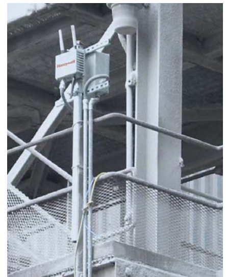
Wiring is a chronic weak point close to a harsh steel furnace.
